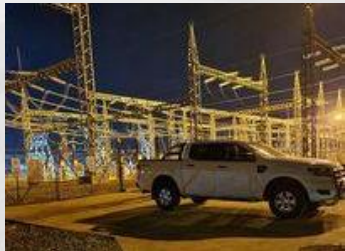
Eskom Substation 12km away
