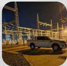
Eskom Substation 12km away
