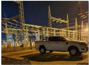
Eskom Substation 12km away
