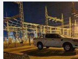
Eskom Substation 12km away
